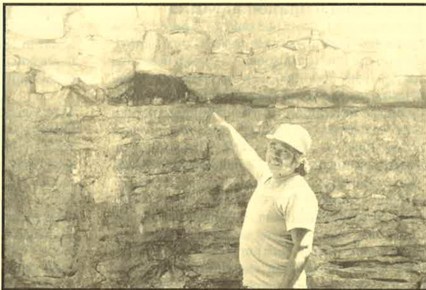
Pete Peynetsa inspects the deteriorating condition of the east wall of the spillway, Upper Nutria Diversion Dam. Photo by F. Bowannie, Jr.
