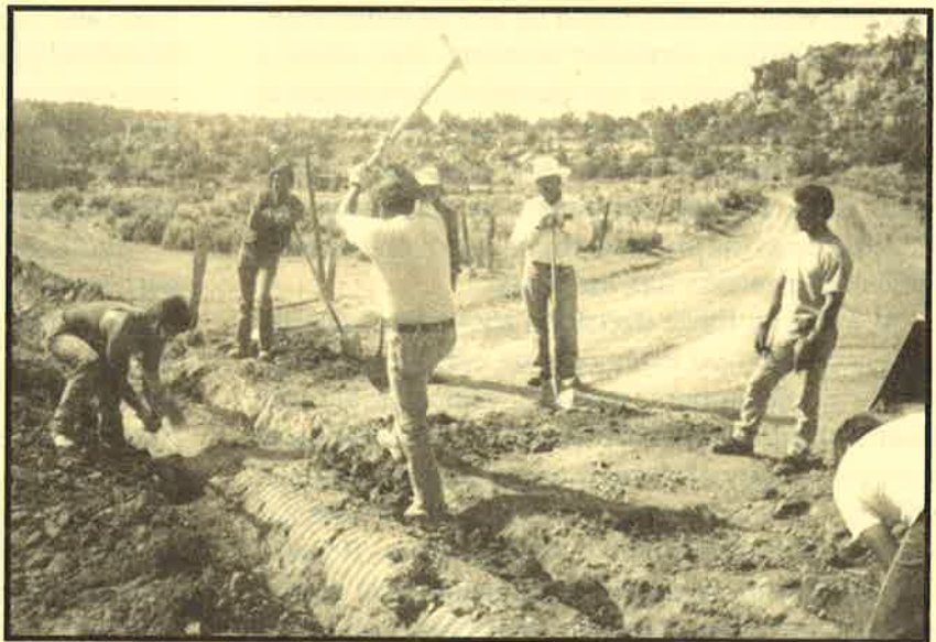
A work party of the Pescado Irrigation Unit repairing a culvert. Photo by D. Eriacho
