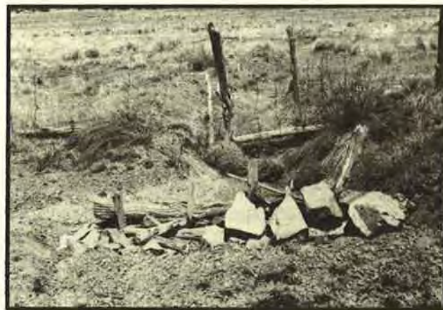
A check dam built by Jones Quam to stop erosion on his rainfed field in Nutria.
