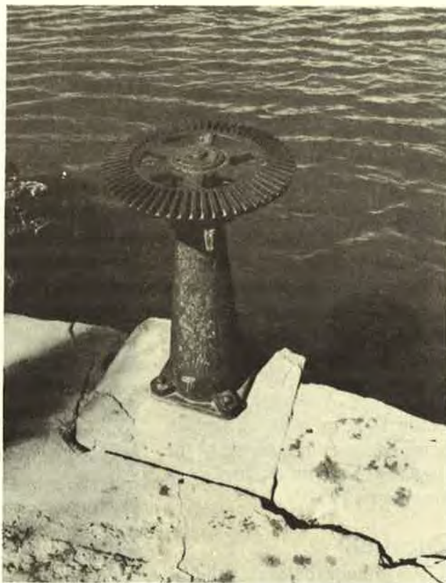
Inoperable Control Gate, Nutria Diversion Dam Spillway. Photo by D. Cleveland
